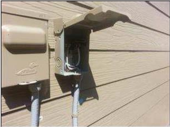
11.5 Item 3(Picture) Condenser shut off
